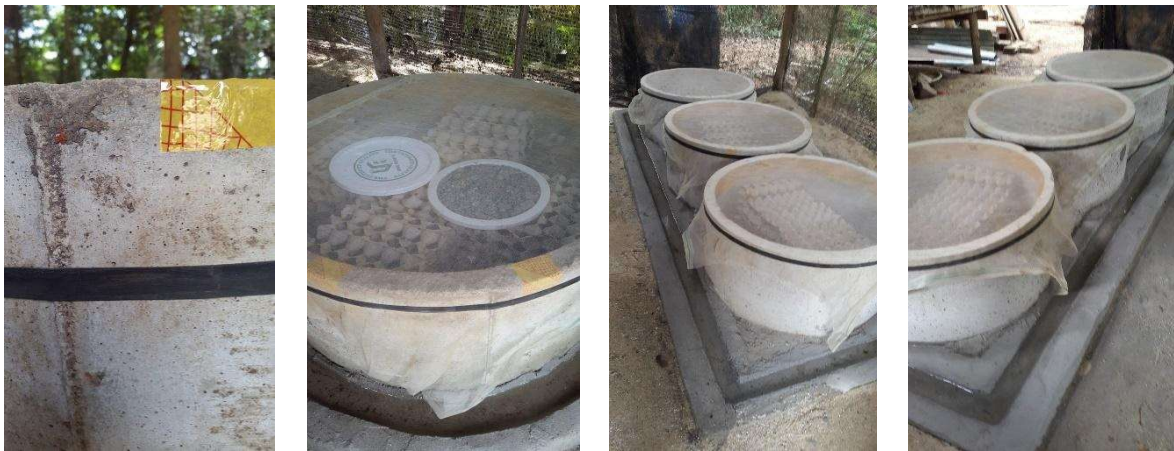
Figure 24: Images on how to cover the tanks tightly with the mesh applying a good pull
